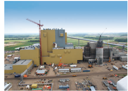
Project Pioneer's generating station, Keephills 3
