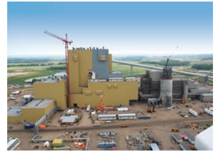
Project Pioneer's generating station, Keephills 3
