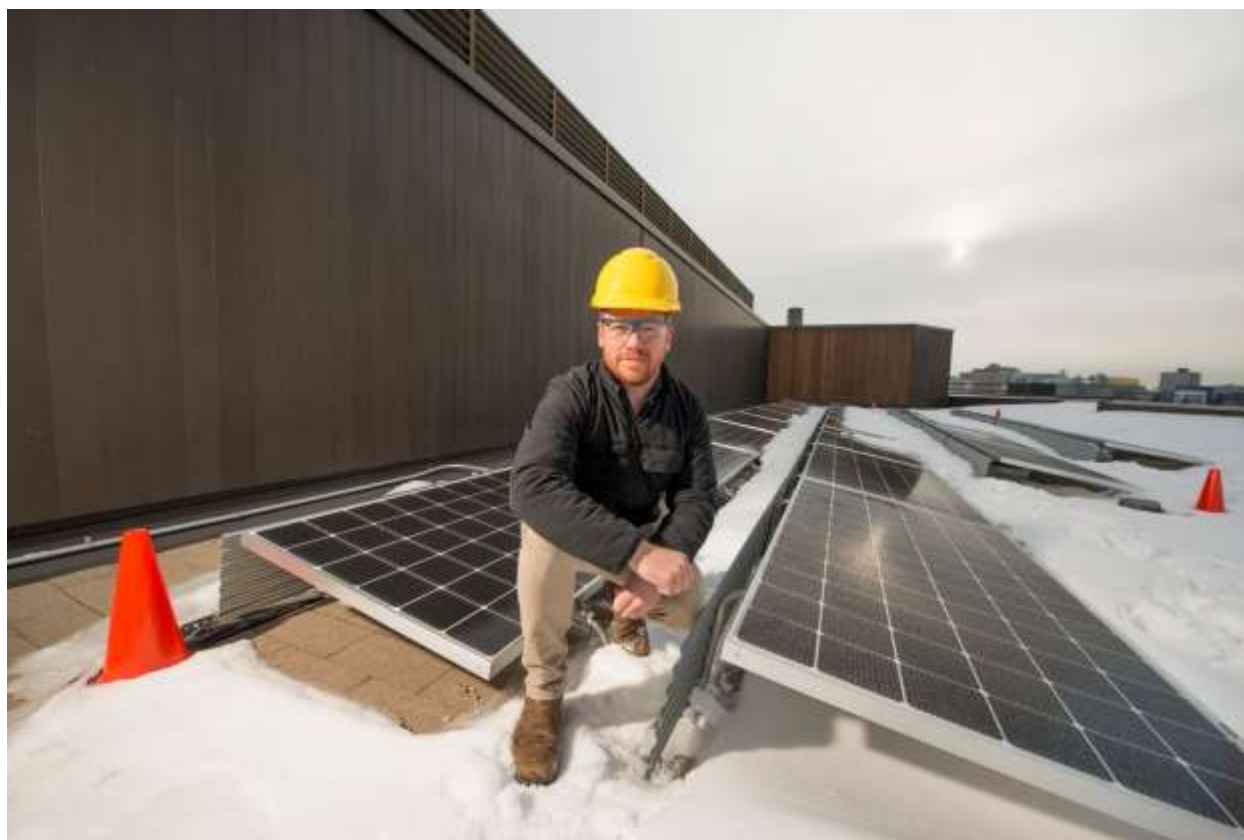
Figure 4 - 10kW Solar installation located on the 3rd floor
