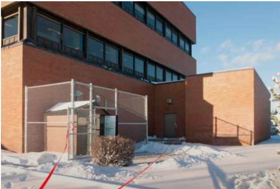
Figure 2 - The battery installation location behind STCC
