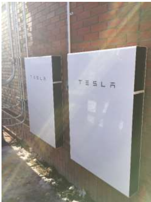
Figure 3 - Tesla Powerwall 2 installation located next to the VRB shed
