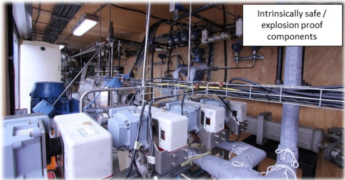
Figure 4.2 Internal View of the Facility
