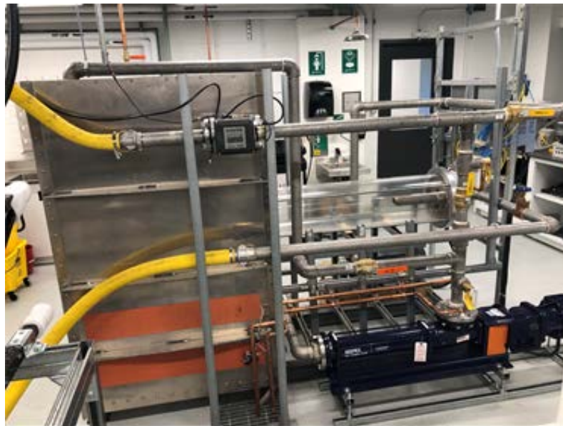
Figure 32 Pumps and reservoir tank.
