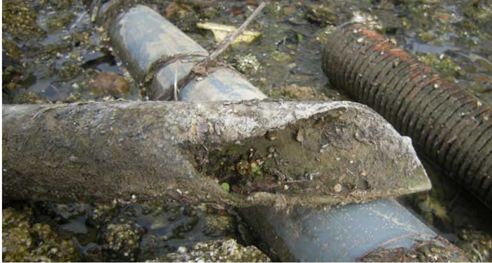
The majority of AC pipes are near the end of their design life.
