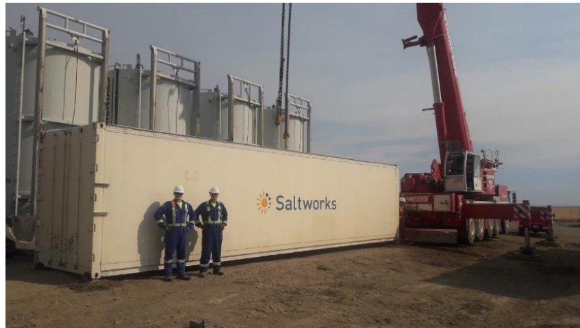
Figure 9: Containerized Flex EDR Organix Pilot Plant
