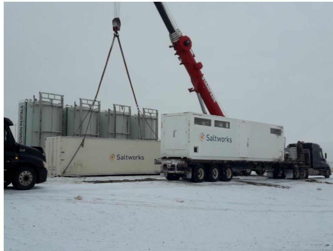
Flex EDR pilot plant at site in southern Alberta, Canada
