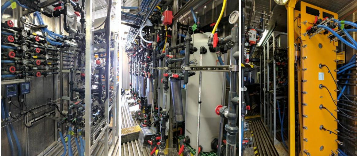
Figure 4. Pilot plant pipework (left), prefiltration (middle), and stack (right)
