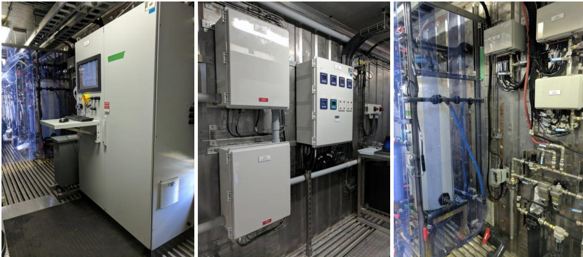
Figure 5. Pilot plant main AC panel (left), control panels (middle), and air system (right)
