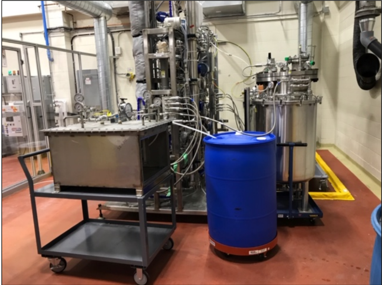
Figure 3: Engineering skid used for some design parameter setting for field unit
