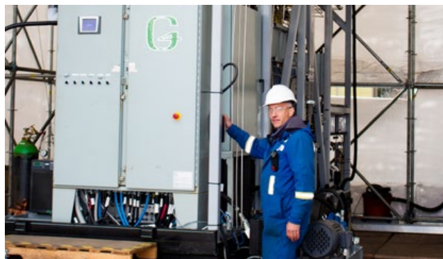
The G4 renewable natural gas unit.
