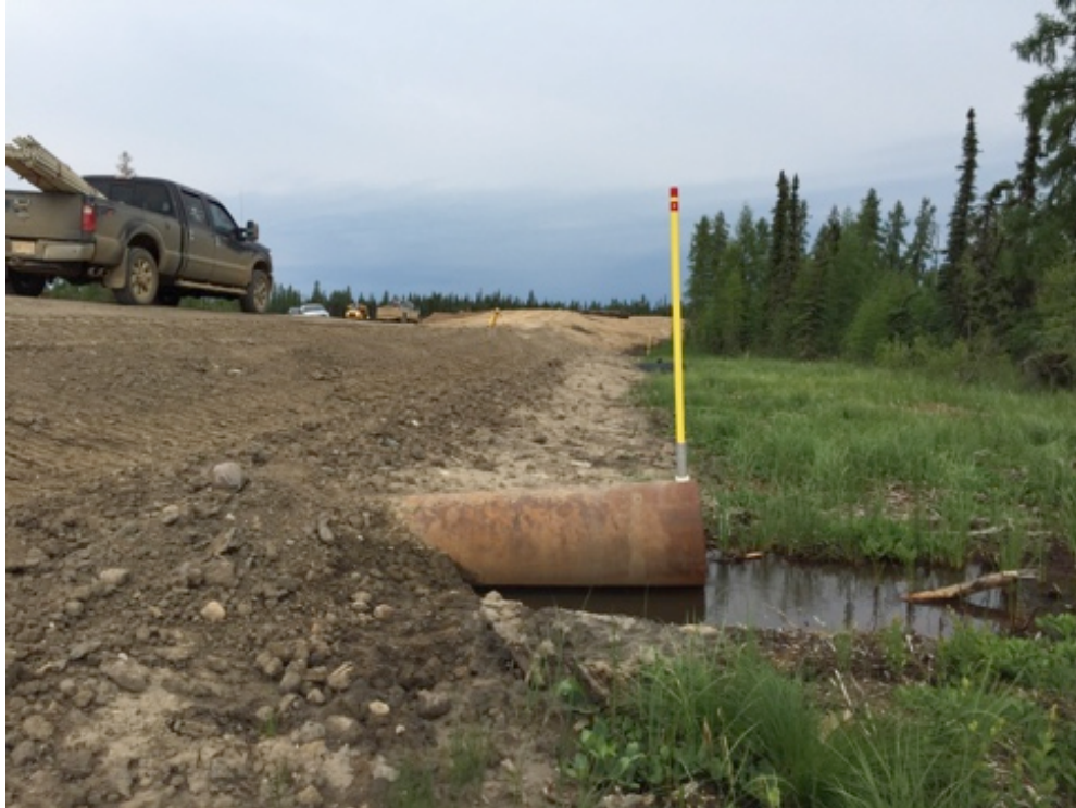
Figure 8. Example of culvert distortion, causing upward deflection of the outlet. Such distortion is common with peatland roads. Corrugated steel culverts are more prone to distortion than steel pipe, like the one pictured.
