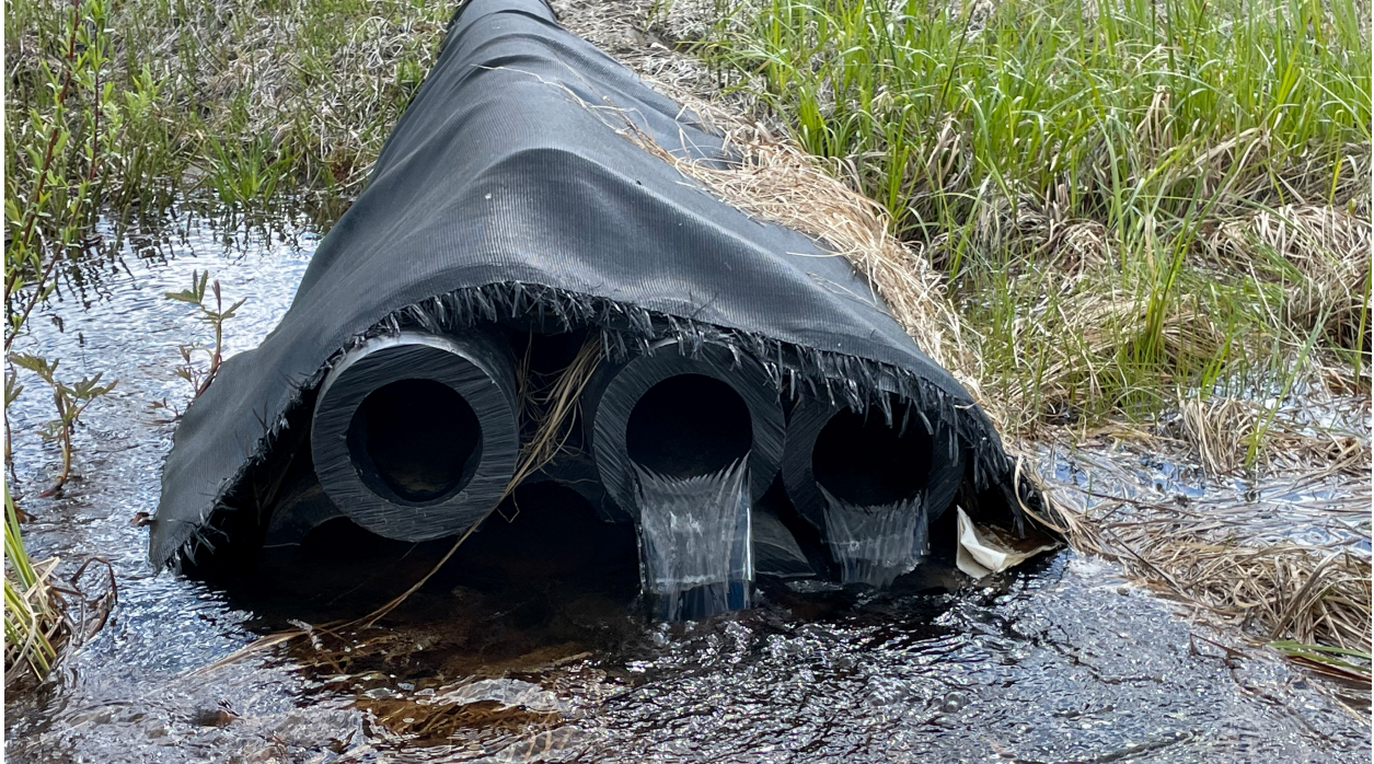
Figure 18. Water flowing out of pipe bundle outlet in late May 2022.
