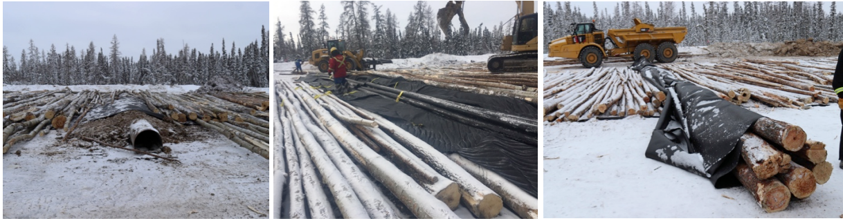
Figure 4. Left: Pre-embedded solid steel culvert covered with mineral fill and abutted with logs. Centre: HDPE pipe bundle being installed among corduroy logs. Right: Log bundle wrapped in a geotextile placed among corduroy logs.
