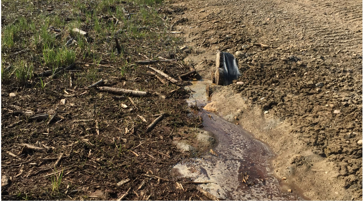
Figure 17. Water along road edge draining into a log bundle during second season post road construction.
