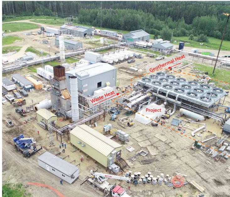
Figure 2 Project plant site with a view of major installed equipment
