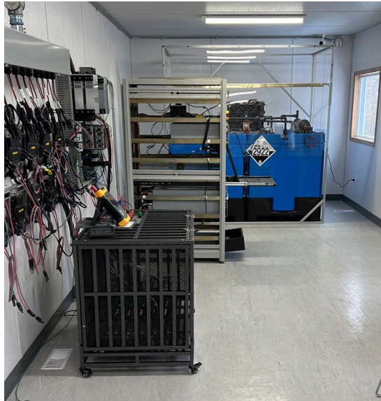
Figure 18. The 5 kW commercial VRFB with power supply and load equipment for charge-discharge battery.
