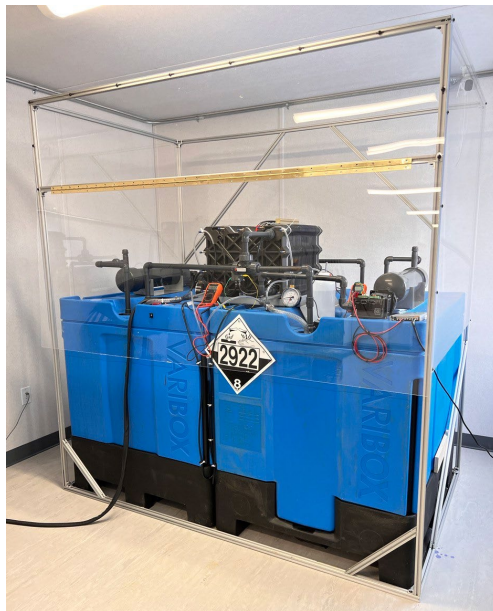
Figure 19. The 5 kW commercial VRFB.
